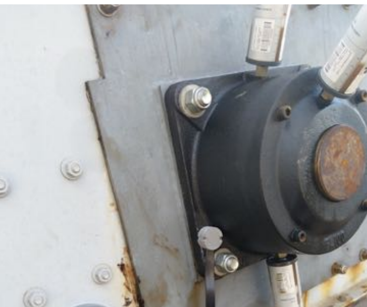
◀ Transport bearing monitoring
