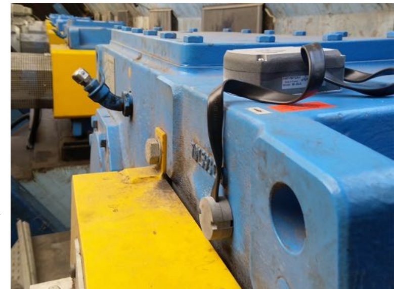
Lift screw gear box monitoring ▶
